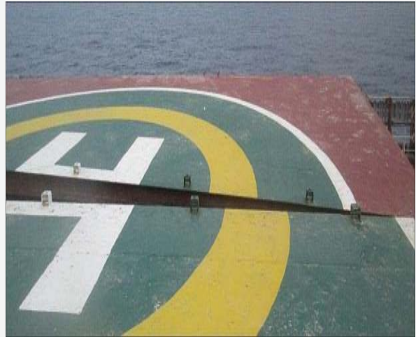
Hatch cove deformed
